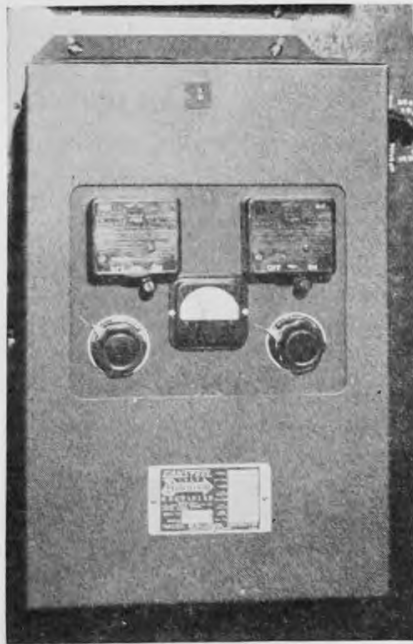
One of the rectifiers for charging batteries in the office
