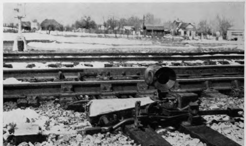
Hand-thrown switch stand with an electric lock
