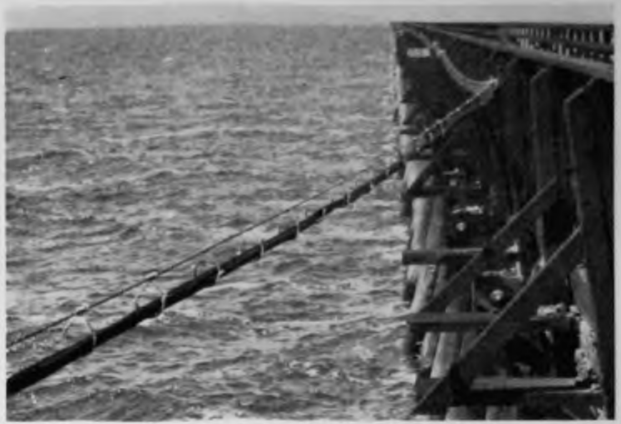
Automatic signal line circuits and a.c. power circuit on the trestle are in cable
