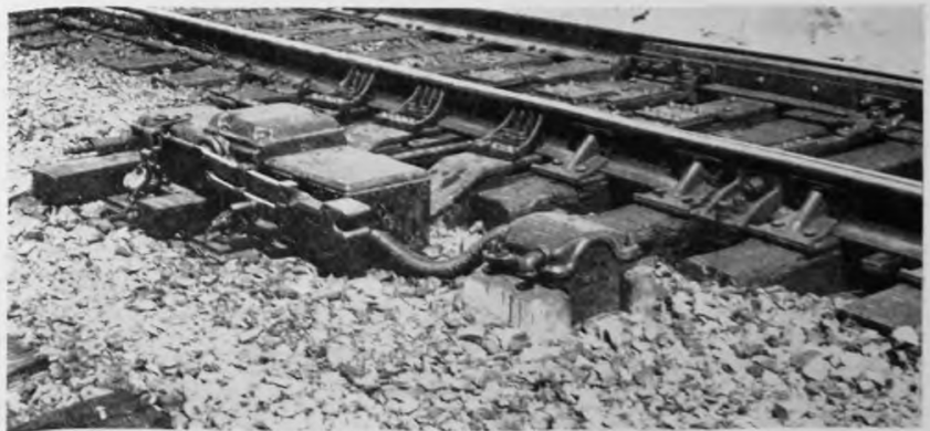
The power switch machines are the dual-control type
