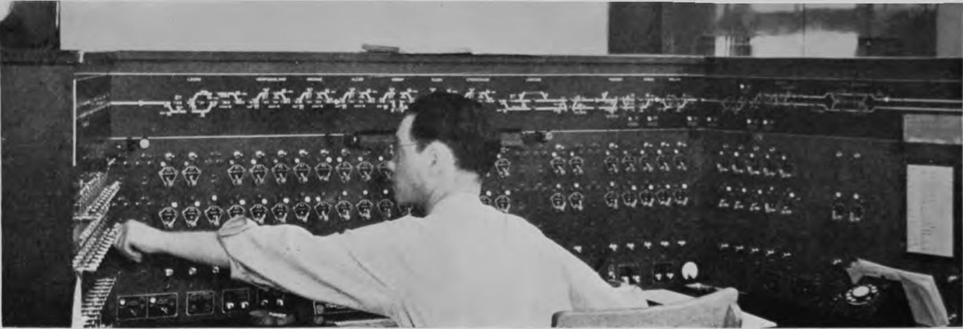
The C.T.C. machine in the office at Ogden, Utah
