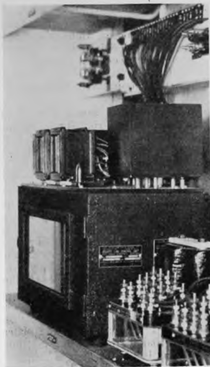
Carrier equipment at Lakeside
