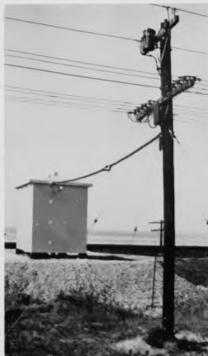
Line transformer on crossarm
