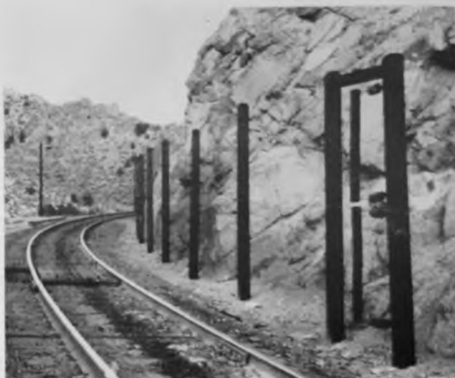
Rock-slide detector fence
