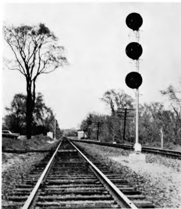
Signals at end of siding
