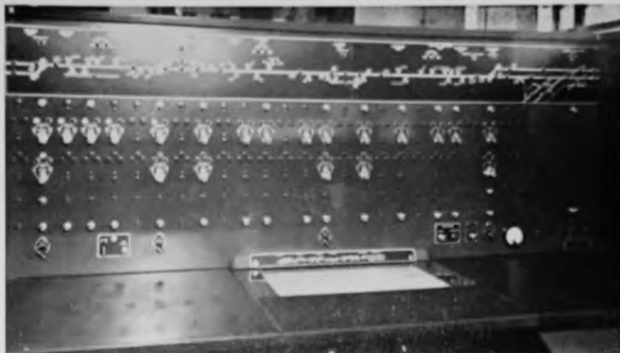
The control machine is in the dispatcher's office at Buffalo
