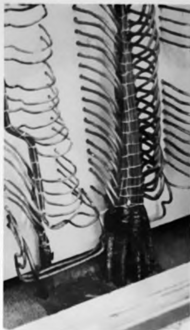
Cable potheads behind board
