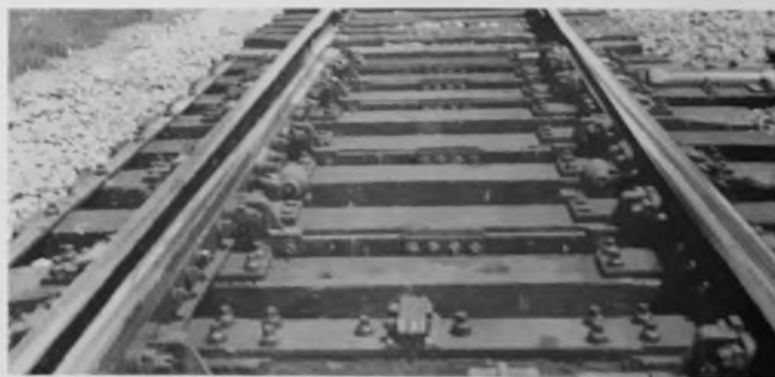
Roller bearings and vertical-pin type rods on switches
