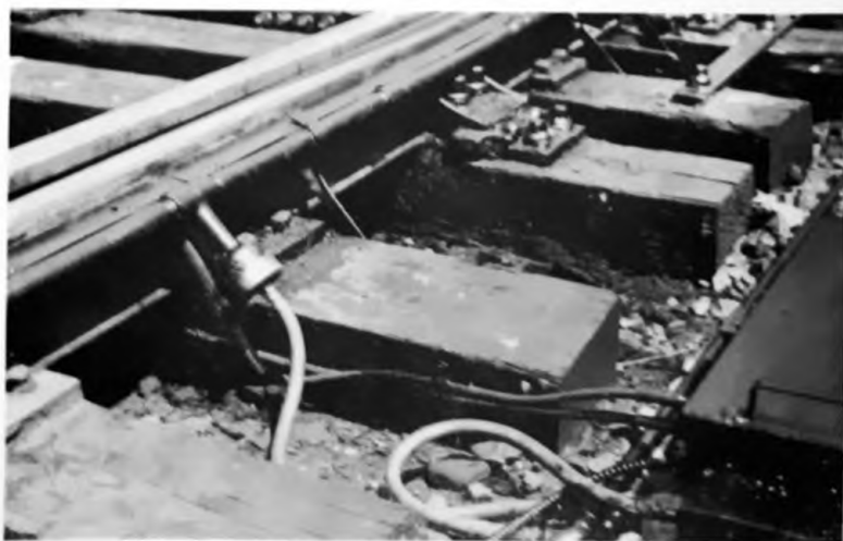
Gas-fired heaters, controlled by dispatcher, melt snow at switches
