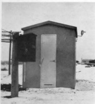
A concrete relay house, with maintainer's call signal and telephone, is located at each control point.
