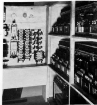
Interior of a concrete relay house showing part of the control equipment and apparatus housed in it.
